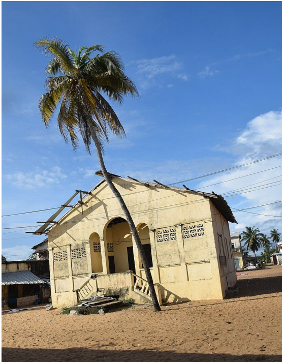
Old building in the historic city of Grand Bassam by User:Adoscam CC-BY-SA-4.0
