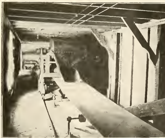
TRIPPER DISCHARGE TO DOCK SPOUT.
