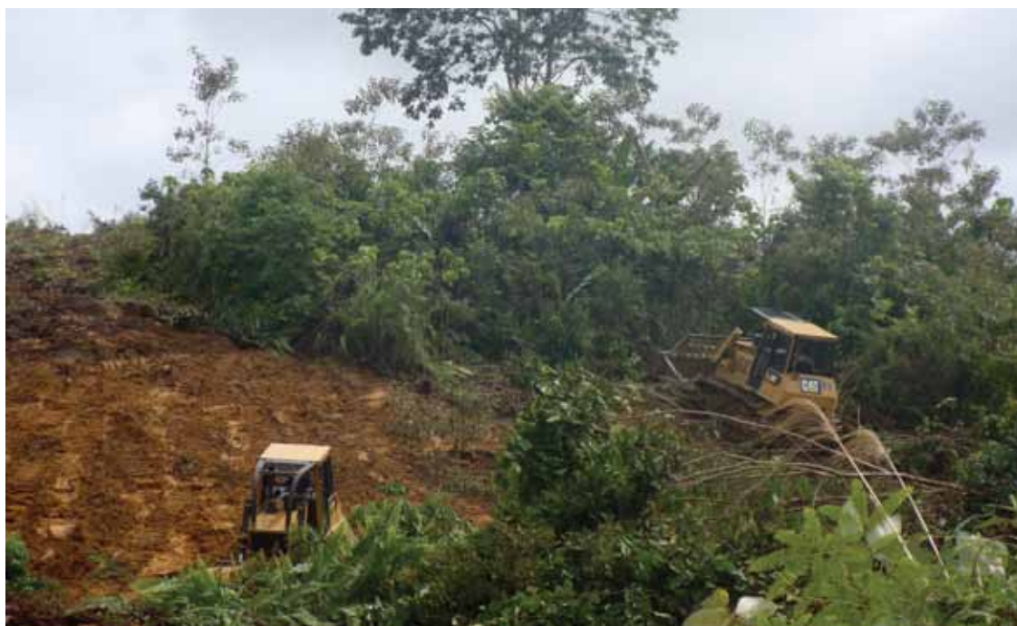
Opening land with bulldozers for establishing a new oil palm plantation. Photo: Stephan Wulffraat
