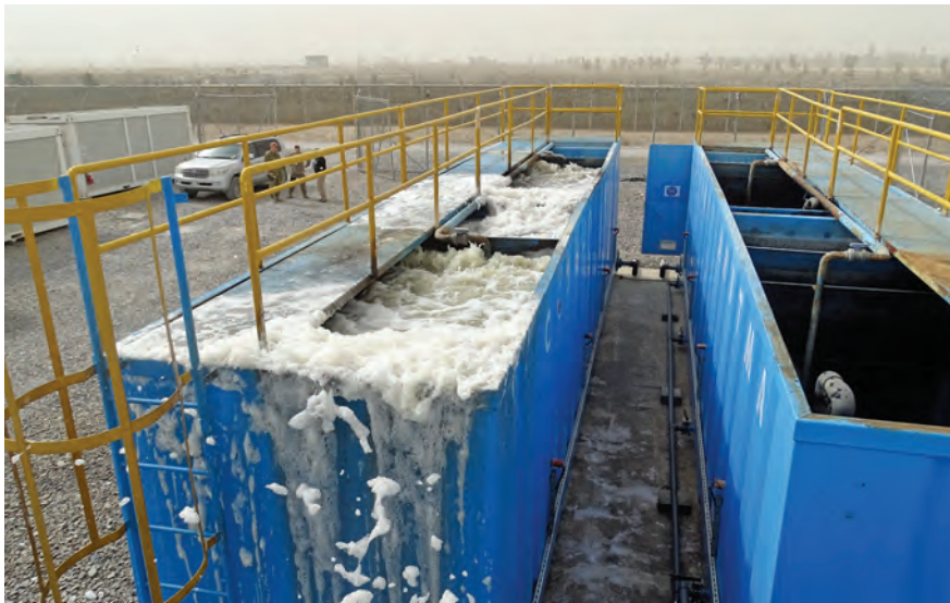
The wastewater treatment plant at the Special Mission Wing facilities at Kandahar Airfield on February 10, 2016, with one nonoperational tank and the other tank overflowing, was examined as part of a SIGAR inspection. (SIGAR photo by Javed Khairandish)
