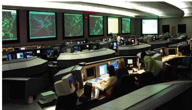
Figure 6-11. An ARTCC Operations Room
