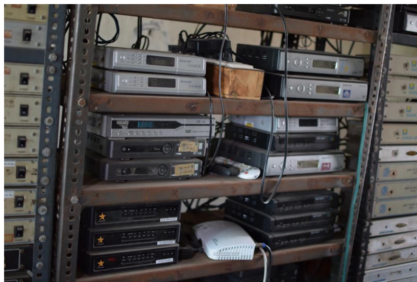
Figure 7: Unused satellite receivers in a control room. Guntur District.
