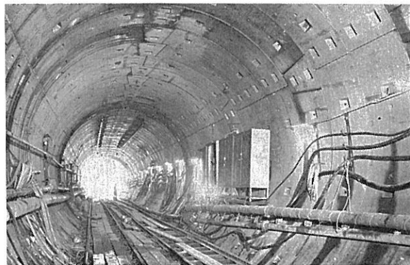
Up track tunnel from Lok Fu to Wong Tai Sin which has been driven under compressed air conditions
