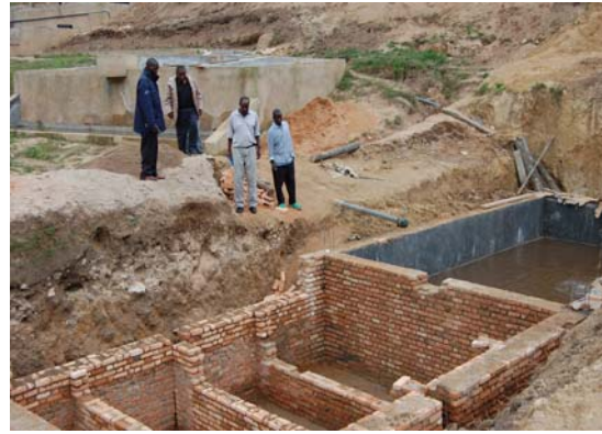
a view of wastewater treatment infrastructure
