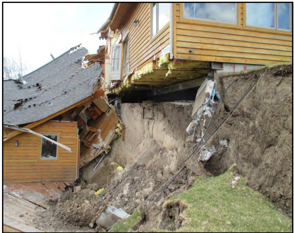
Figure 20: Headscarp of the landslide directly under the inside edge of the southeastern foundation of the house at 1045 Budge Drive
