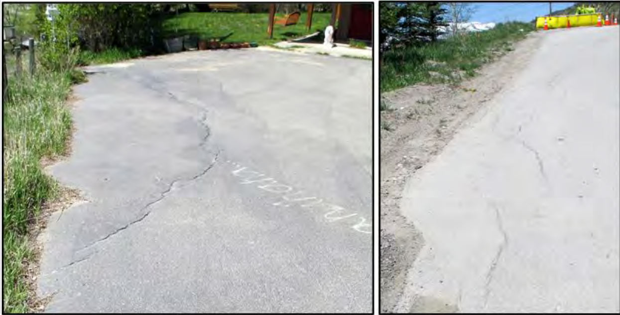
Figure 15: Crack in the driveway at 980 Budge Drive (left) and just to the north along Budge Drive (right) that were first observed in 2009 shortly after a malfunction of the sprinkler system for the condominiums at 981 Budge Drive caused considerable water to flow down the hill. Views looking west.
