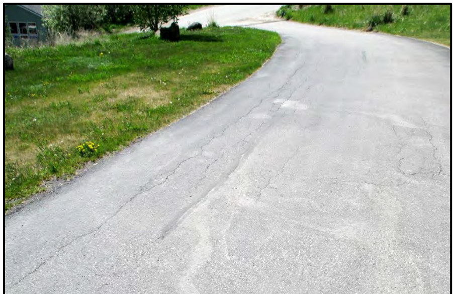
Figure 16: Cracks in the driveway to the condominiums at 981 Budge Drive, looking west.
