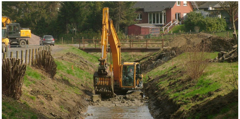
Renaturation of the Emscher system: Demolition of concrete borders in the Rüpingsbach in Dortmund-Schönau (Photo by Stefan Kunzmann)
