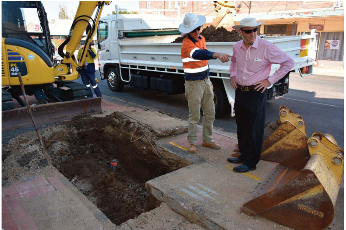
Work has commenced to remove up to 19 underground fuels tanks from Bradley Street
