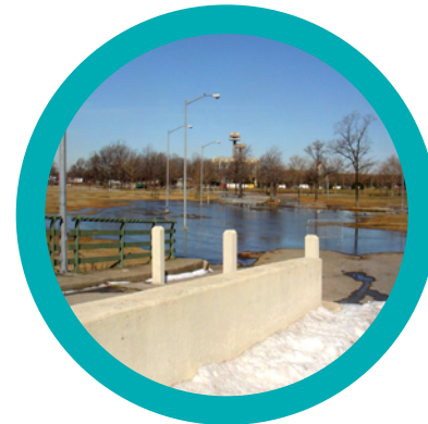
Major Areas of Poor Drainage
