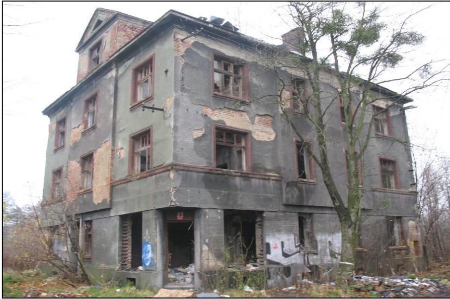
Figure 22 Dilapidated building in Hrušov - north eastern part
