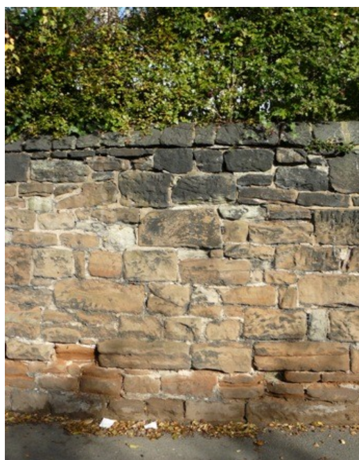
Figure 33 A sandstone retaining wall on (what is now the southern end of) Powell Street, believed to originate in the first half of the nineteenth century
