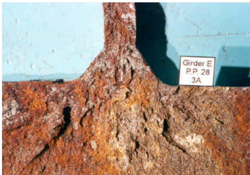
Figure 65: Cleavage Fracture in the Web-Flange Area of the Bottom Flange of Girder E P.P. 28
