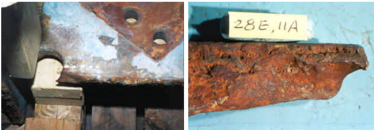
Figure 68: Girder E P.P. 28 Shelf Plate Showing the Hole Repair and Crack Surface Adjacent to the Hole
