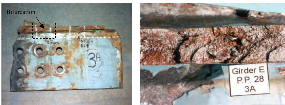
Figure 66: Crack Bifurcation in the Web of Girder E P.P. 28 Near the Fracture Origin.
