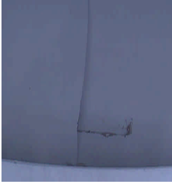
Figure 5: Cracked Web of Girder D-28
