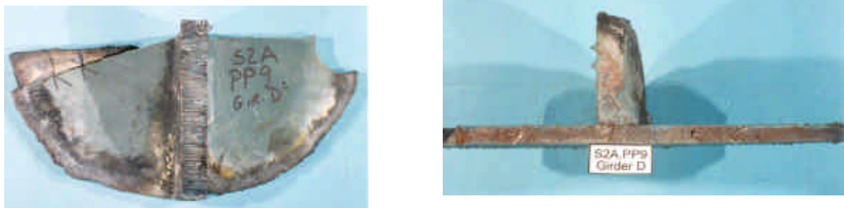
Figure 57: Web Crack Removed From Girder D at P.P. 9 at the Shelf Plate Connection
