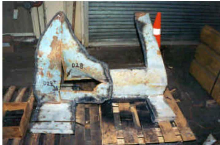
Figure 52: Section of Girder D P.P. 28 Containing the Crack Origin Area and Arrested Crack in the Bottom Flange
