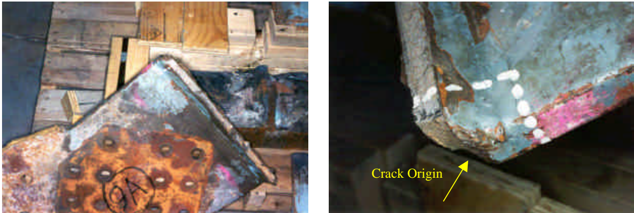
Figure 48: Shelf Plate With Web Fracture Origin at the Weld Termination. (Girder E P.P. 28)
