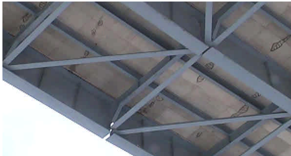
Figure 4: Visible Fractures of Center Girder E-28 and East Girder F-28
